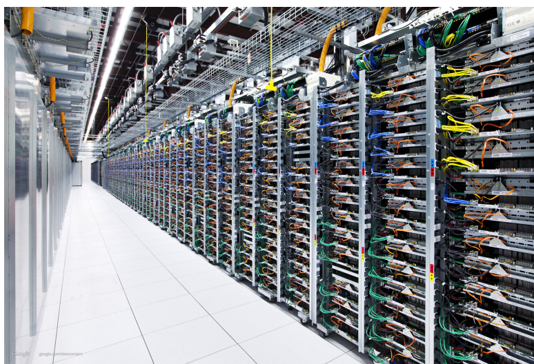
Figure 1.1: TierPoint datacenters, Dallas [1].
